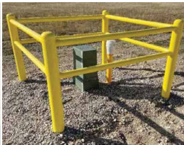
Above-grade enclosures of AC mitigation PCR and RMU.
