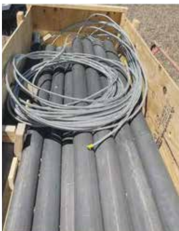
Graphite anodes ready for installation.
